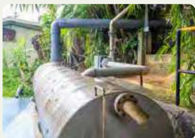
Backwash water recovery project in the Water Treatment Plant
