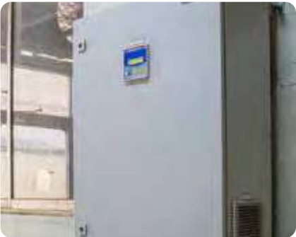
Energy monitoring system implementation
