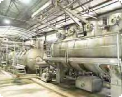
Increased the Cooling water recovery in the Dye house department
