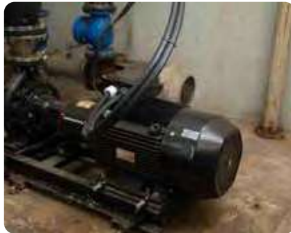
Energy efficient pump replacement at the wastewater treatment plant and effluent treatment plant
