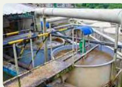
Efficiency improvement of Chemical mixing system
