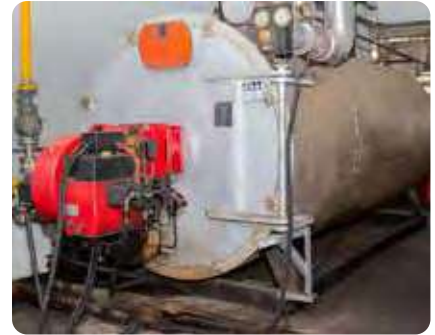
New Thermic oil replacement of TB 01 and TB 06 thermic heater lines system
