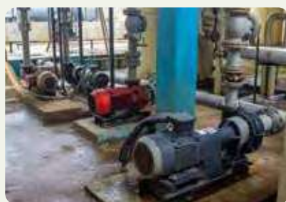
Water sump level controlling automation system and automation of River water pumps
